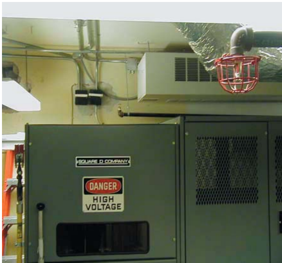
Figure 1: Sprinkler installed above electrical closet
