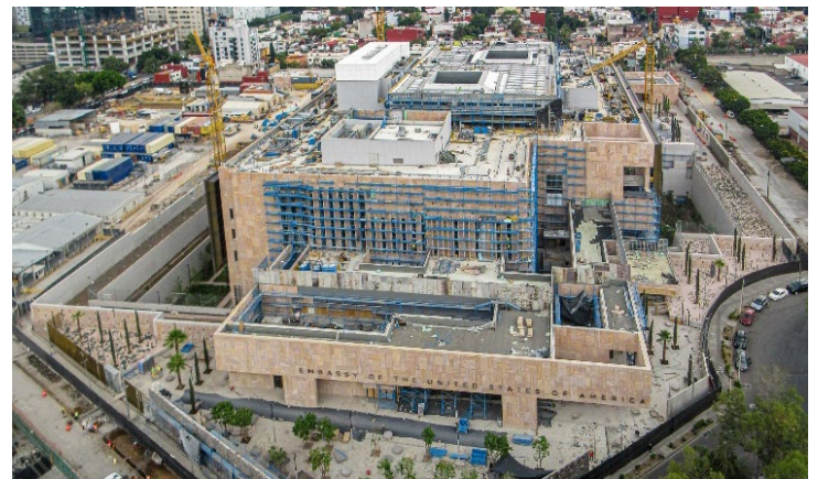
An aerial view showcases the construction progress of the new U.S. embassy building in Mexico City. Photo courtesy of Embassy Mexico City.
