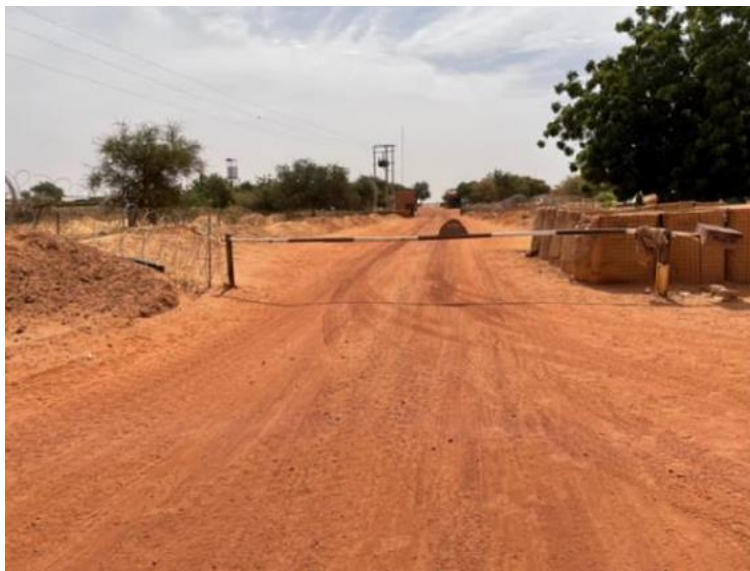
Figure 7: Example of incomplete contract work. The work at a site in Niger was reported as 80 percent complete. However, many tasks were left unfinished, such as constructing an entry control point where nothing had been done. (Source: Bureau of Administration.)
